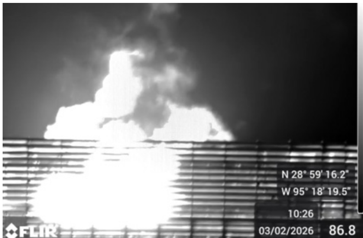
Optical Gas Imaging Footage of the flare at the Pretreatment Plant taken by Jack McDonald. The gray plume indicates uncombusted hydrocarbons.
